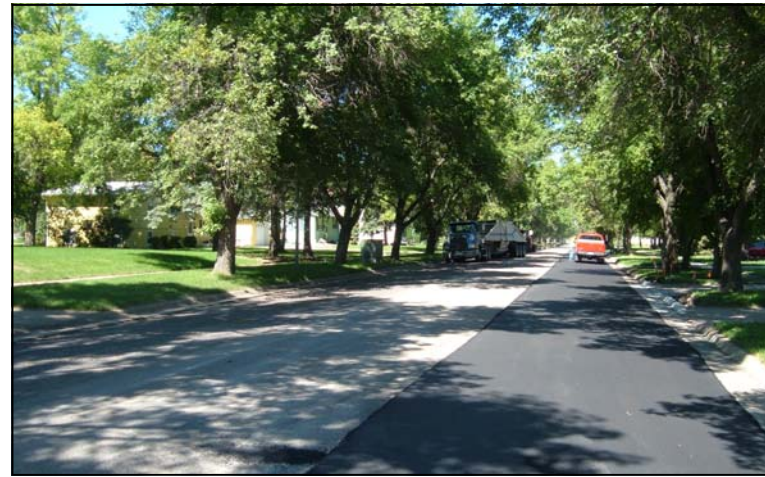
The difference is clear on this section of roadway where half of the street has already been overlaid with new asphalt.
