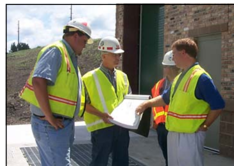
Greg Boppre and the Corps review plans for the flood protection project, 2003.
