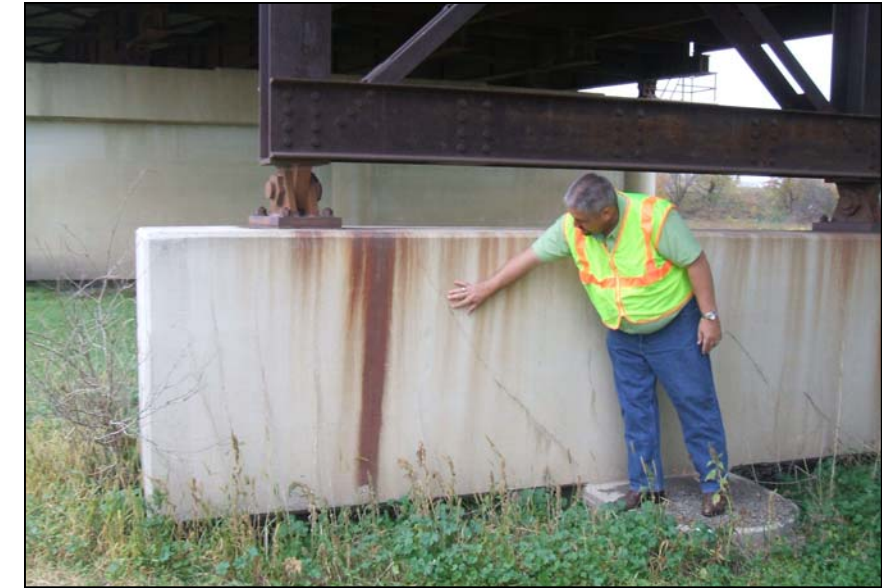
Brad Bail examines a minor surface crack in one of the foundations for the Louis Murray bridge.
