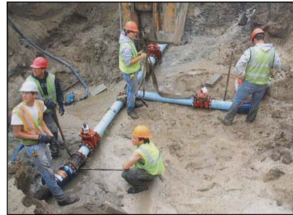
Construction workers install an extension (light blue pipe) to the existing watermain (dark pipe in lower right corner) in Greenbush as part of the water system improvements project.
